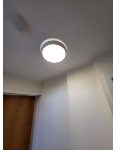
Lighting (Standard and Emergency Lights)
